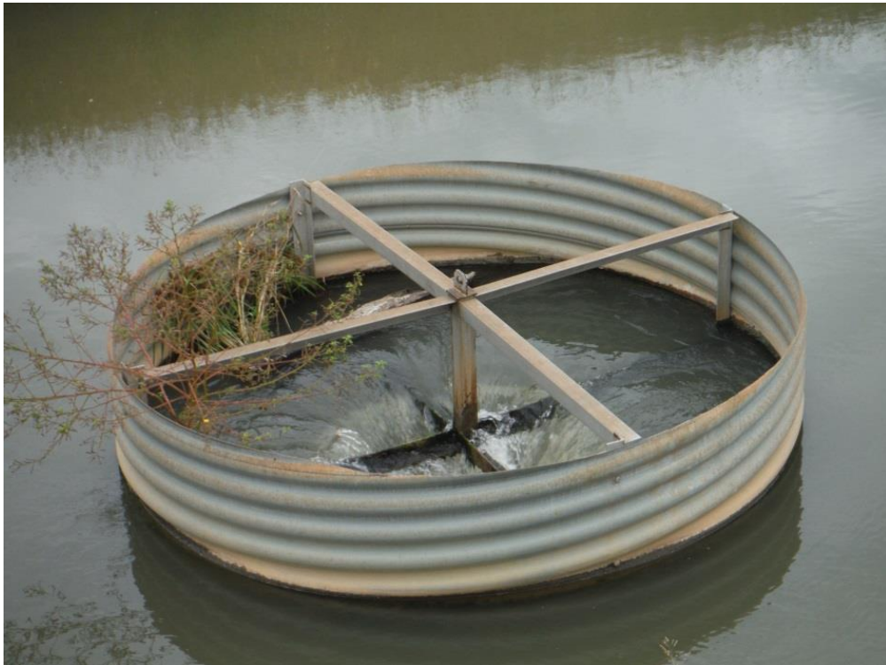
Photo 14 – Slag Stilling Pond 2C spillway skimmer, south
