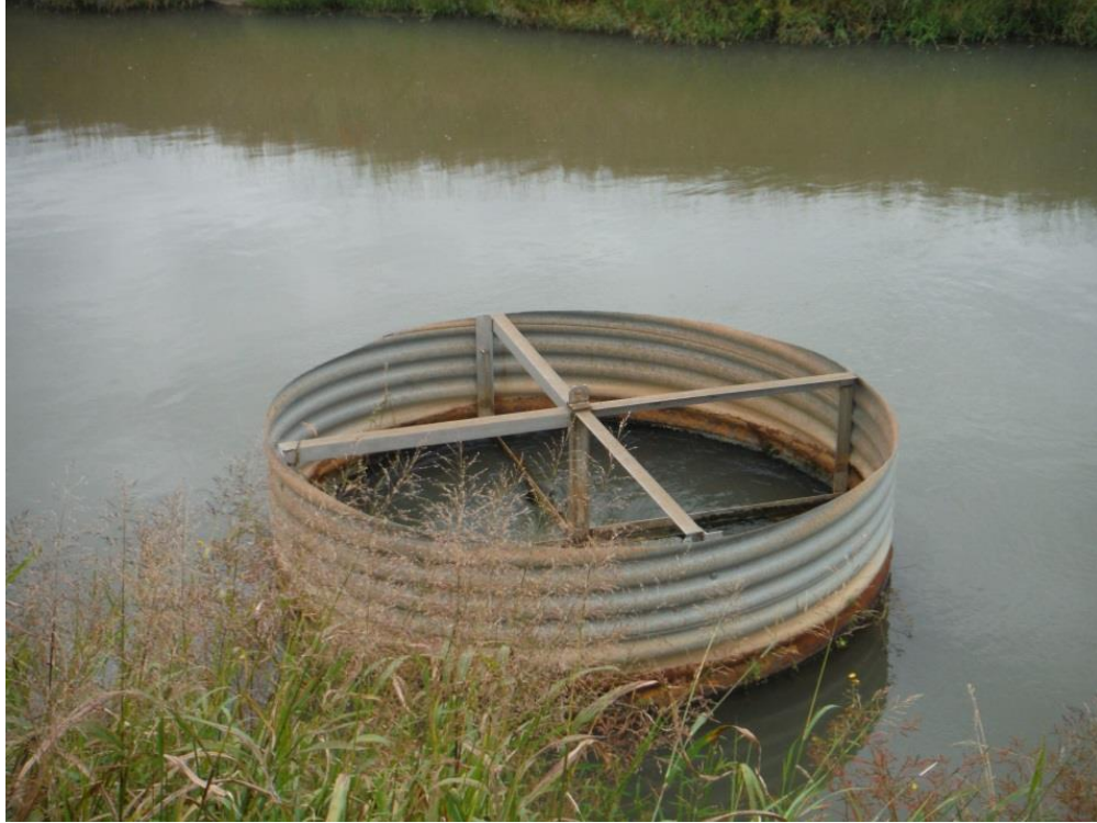
Photo 13 – Slag Stilling Pond 2C spillway skimmer, middle
