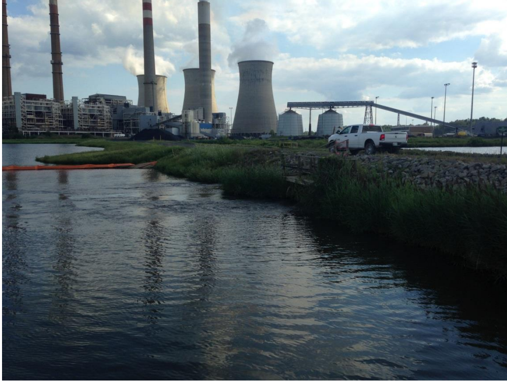
Photo 3 –Slag Pond 2A & 2B splitter dike condition, east side
