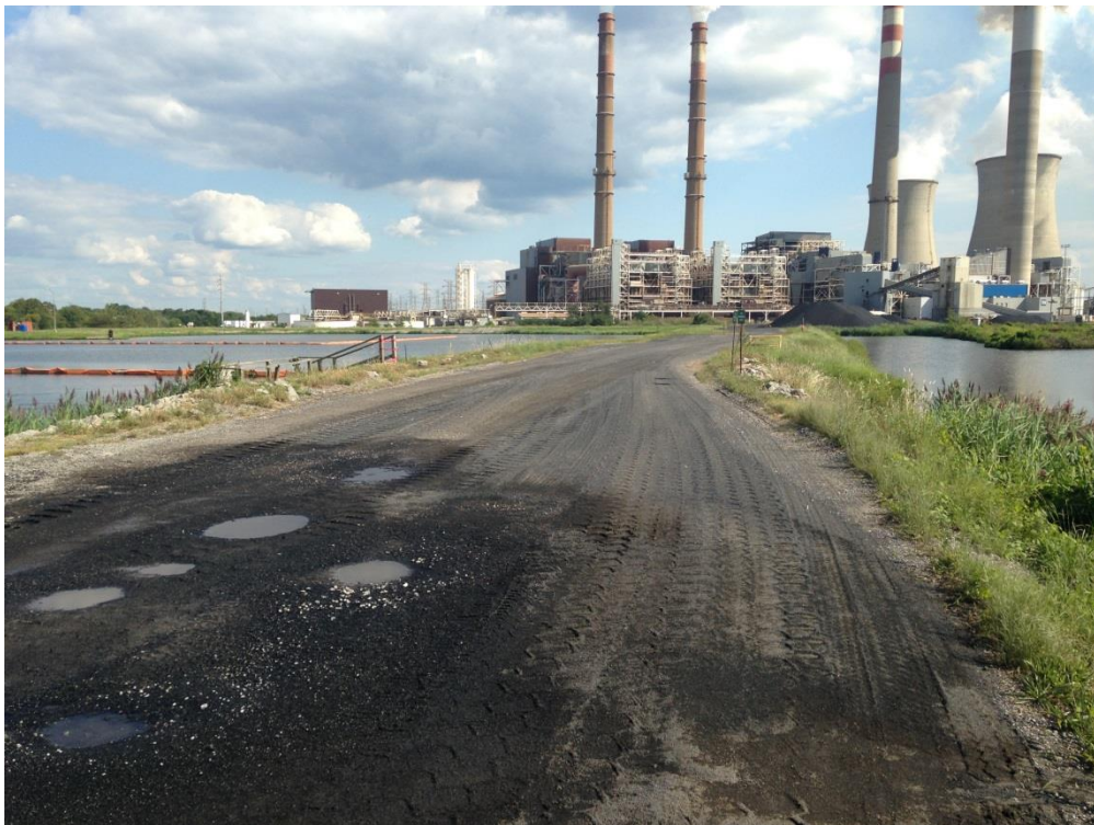
Photo 2 – Slag Pond 2A & 2B splitter dike condition, top
