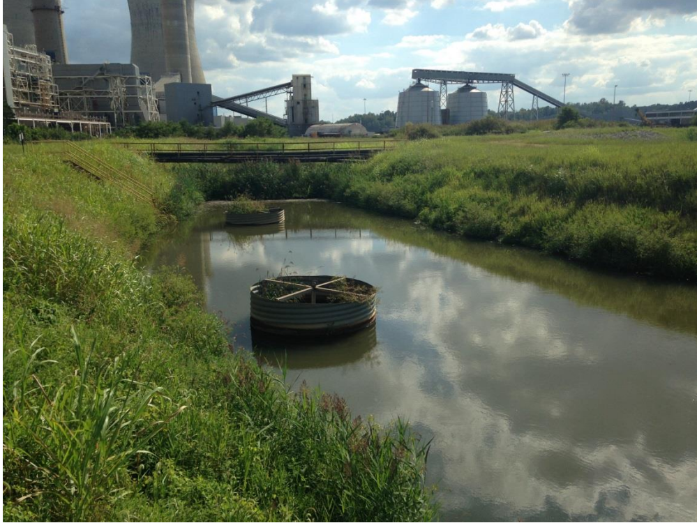
Photo 11 –Slag Stilling Pond 2C dike conditions
