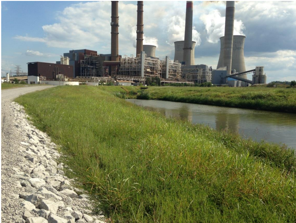
Photo 10 – Slag Stilling Pond 2C dike conditions
