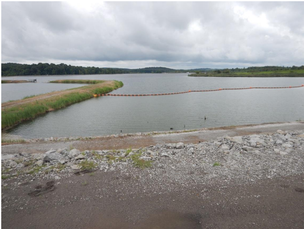
Photo 8 – North dike condition
