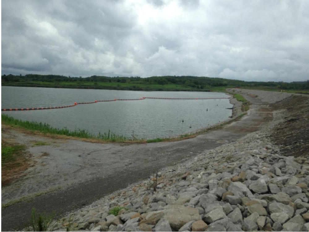
Photo 9 – North dike condition
