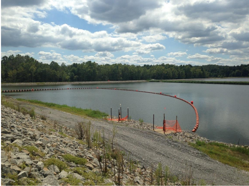
Photo 7 – North dike condition
