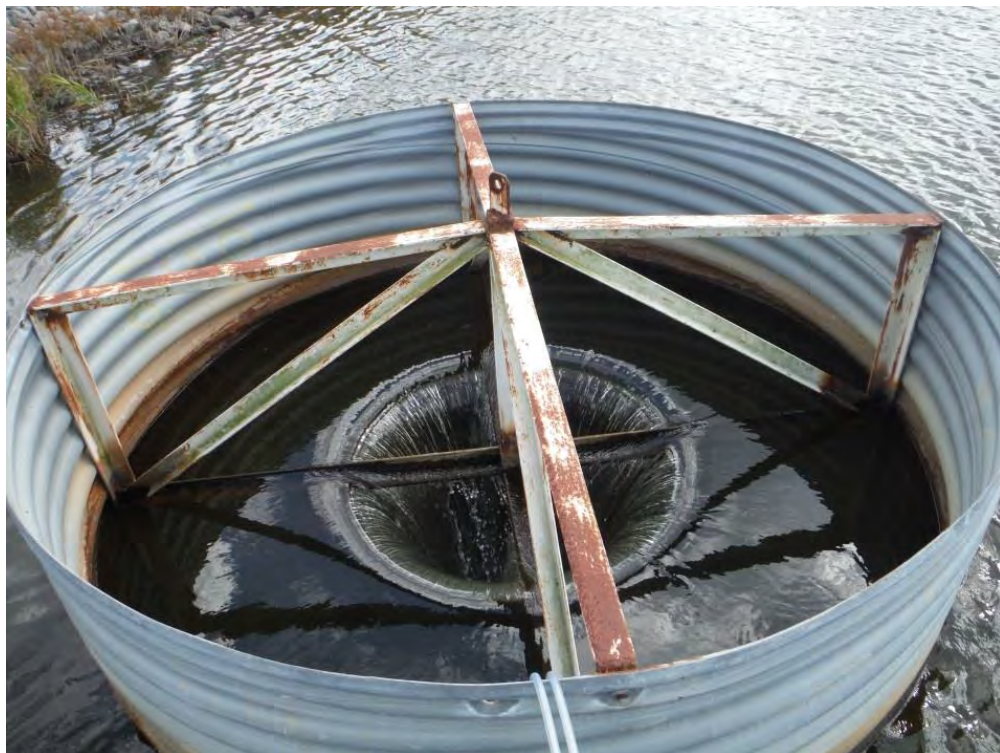
Photo 12 – Spillway skimmer, middle (Typ.)
