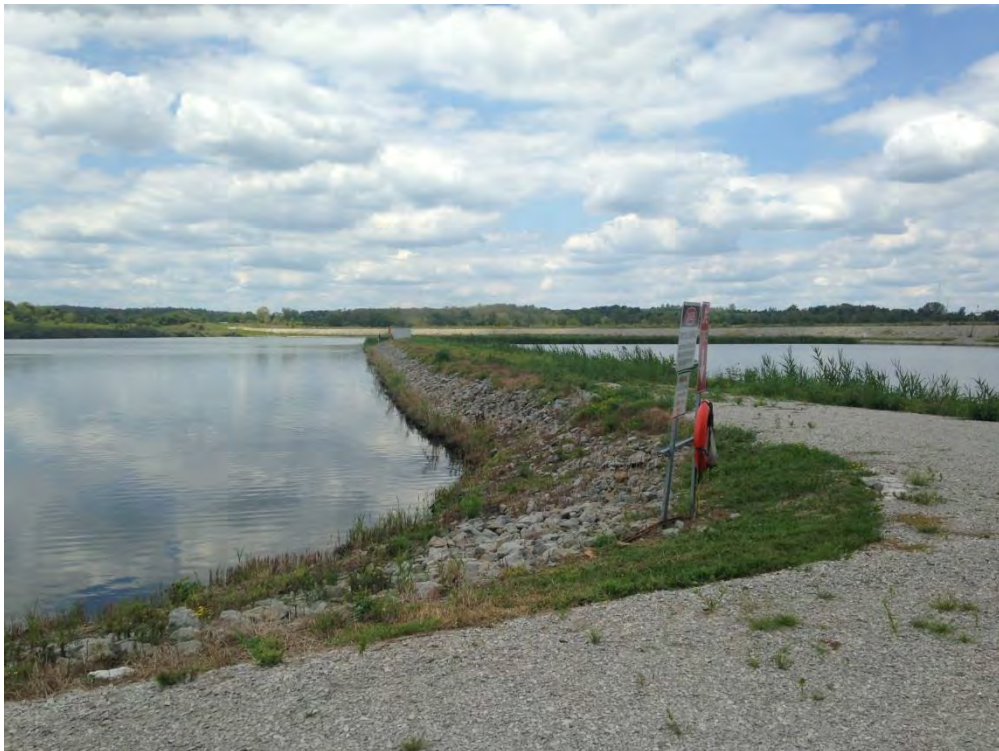
Photo 4 – Stilling Pond dike condition
