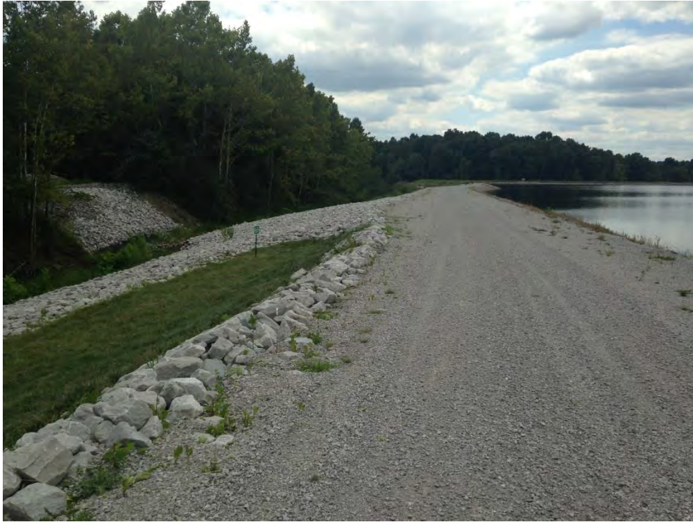
Photo 3 – East dike condition
