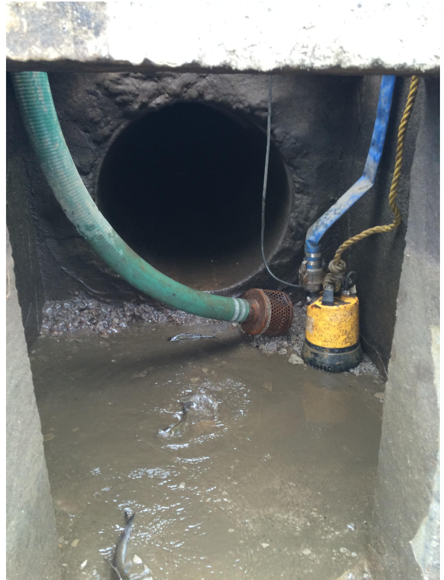
Picture 2: Typical condition of pipe inlets at spillway junction box during construction of Ash Pond Lowering and Flow Diversion Project (2016)
