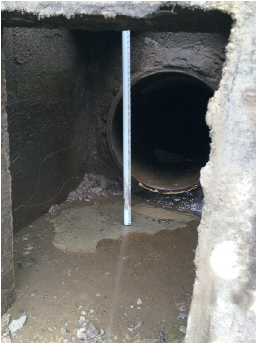
Picture 1: Typical condition of pipe inlets at spillway junction box during construction of Ash Pond Lowering and Flow Diversion Project (2016)
