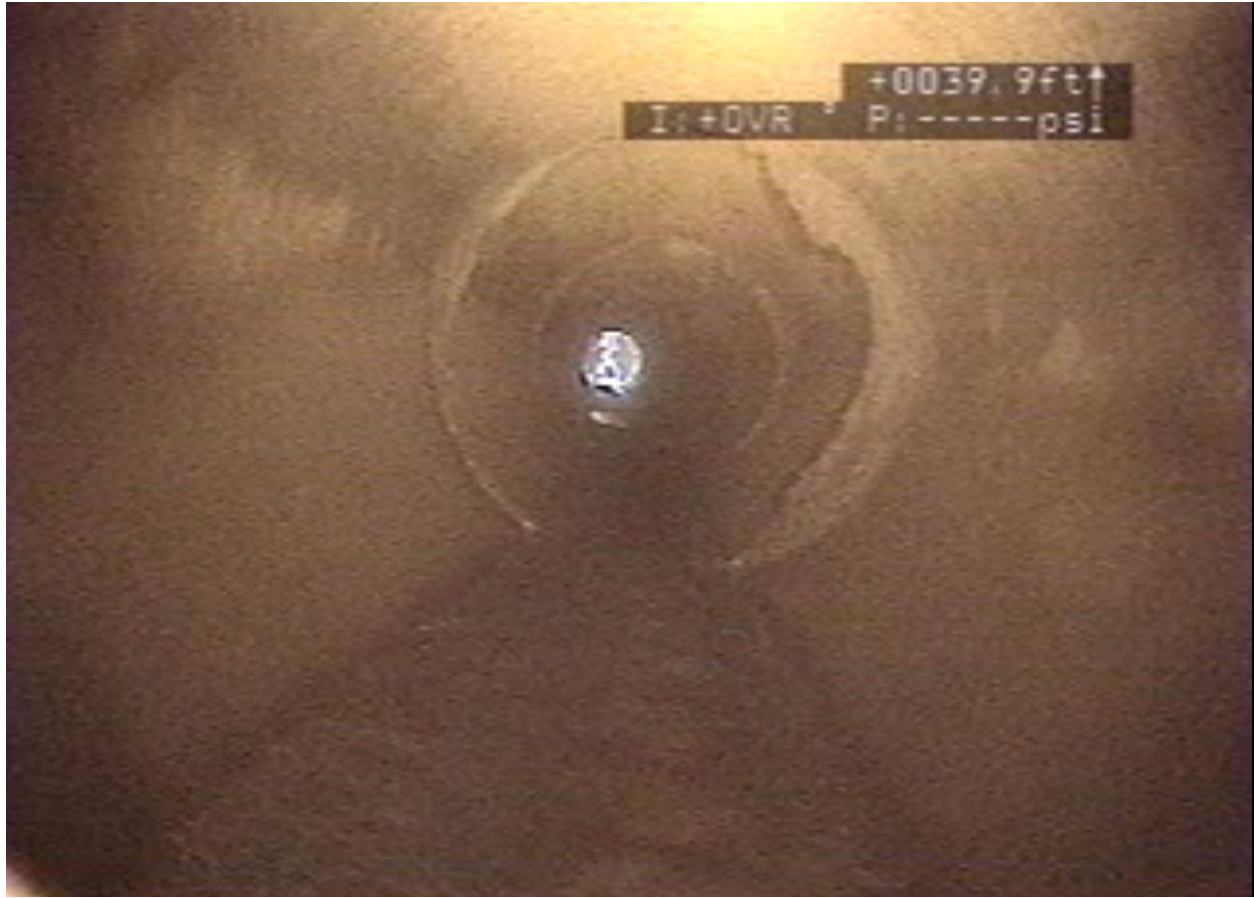
Image 1. Video inspection of outlet pipe from middle riser in Stilling Pond 2C, view looking towards spillway riser showing minor encrustation and minimal leaking.
