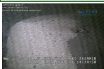
305 ft from manway 17 sand deposit ontop of silt. C1.jpg
