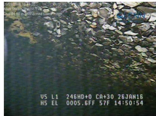
Figure 3 – 800' downstream from manhole No. 17. Example of exposed aggregate with loose cement paste.
