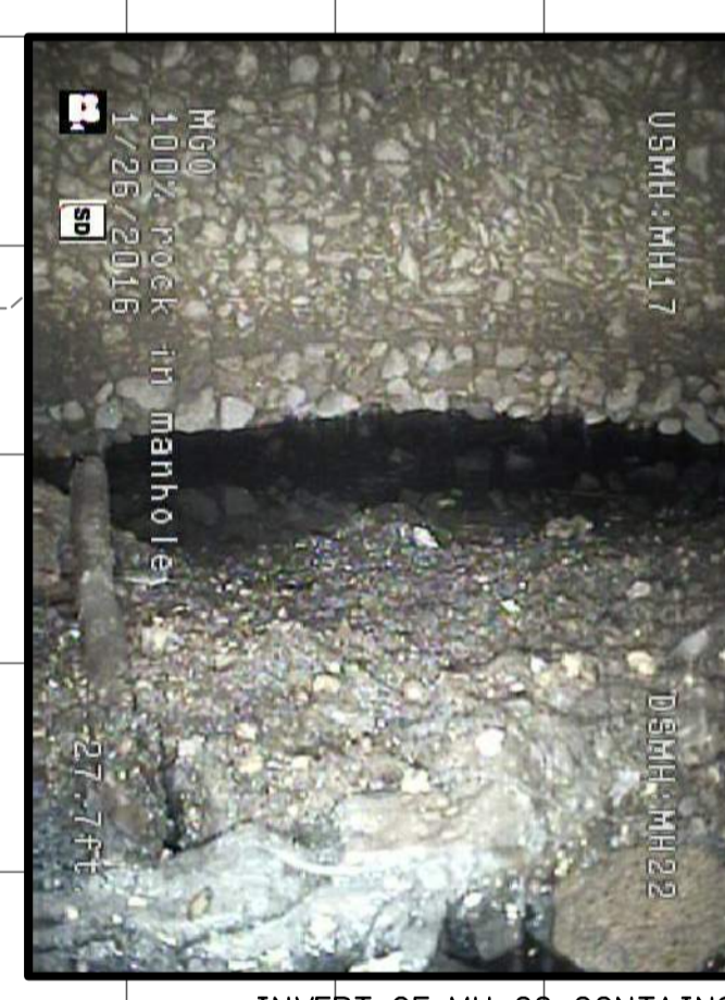
INVERT OF MH 22 CONTAINS APPROX. 95% SEDIMENT
