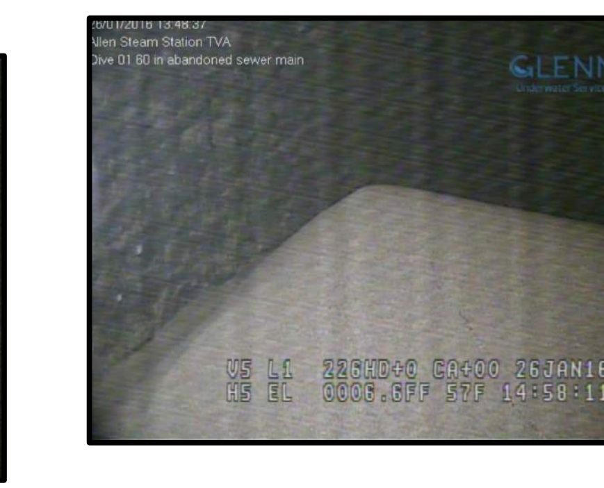
STA. 28+10 SEDIMENT DEPOSIT IN A CONE SHAPE AT INVERT OF RADIAL JOINT
