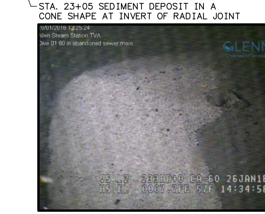
STA. 23+05 SEDIMENT DEPOSIT IN A CONE SHAPE AT INVERT OF RADIAL JOINT
