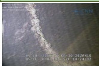
213 ft from manway 17 view of joint with material_C1.jpg
