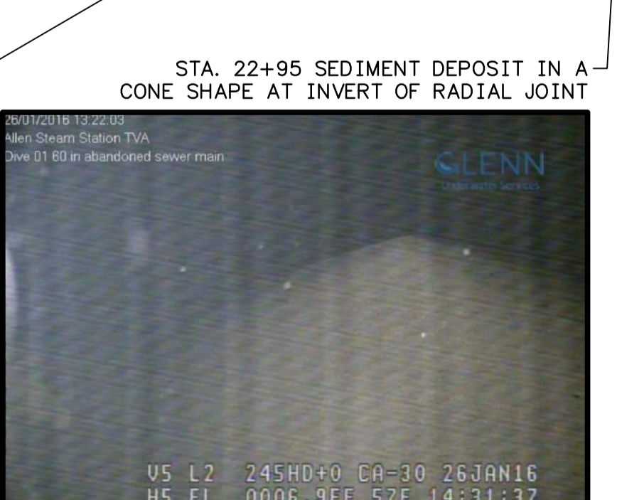
STA. 22+95 SEDIMENT DEPOSIT IN A CONE SHAPE AT INVERT OF RADIAL JOINT
