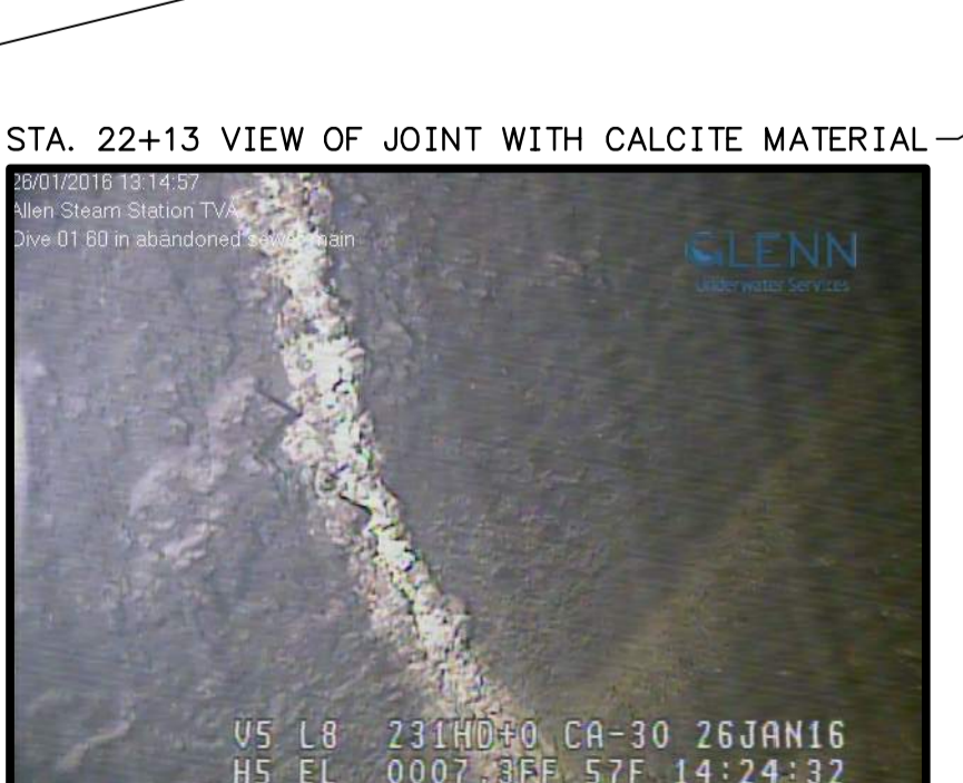
STA. 22+13 VIEW OF JOINT WITH CALCITE MATERIAL
