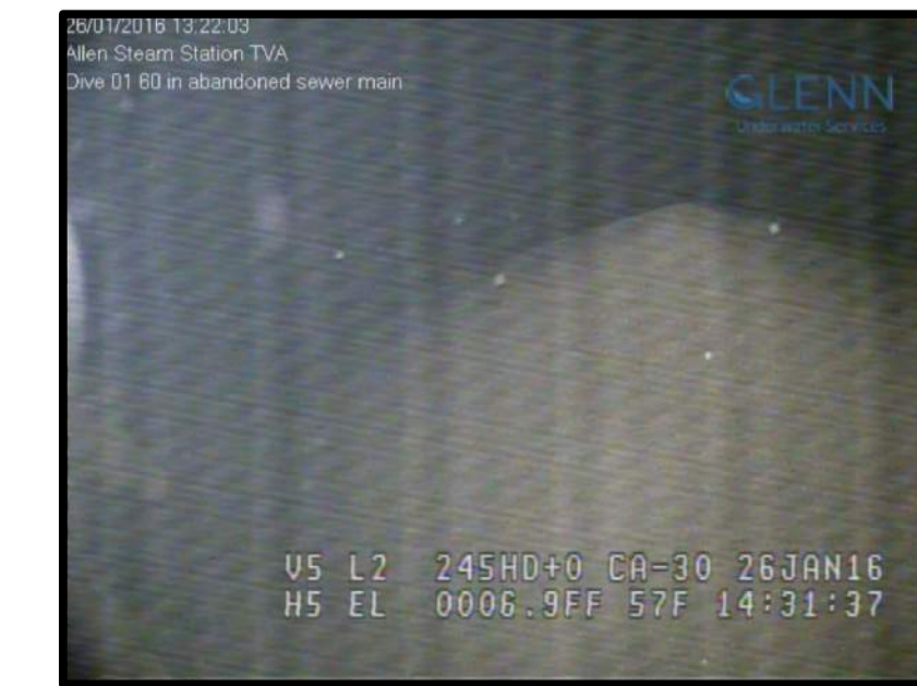
STA. 22+95 SEDIMENT DEPOSIT IN A CONE SHAPE AT INVERT OF RADIAL JOINT
