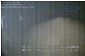
295 ft from manway 17. Sand deposit at invert of pipe. below joint. C1.jpg
