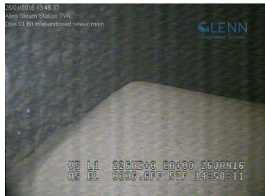
Figure 1 – 810' from manhole No. 17. Fine sand deposit at invert of pipe.
