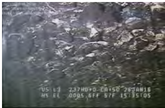
1390 ft from manway 17 exposed aggregate at crown of pipe C1.jpg
