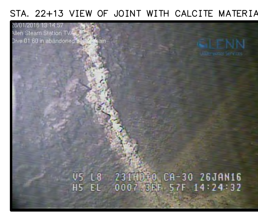
STA. 22+13 VIEW OF JOINT WITH CALCITE MATERIAL
