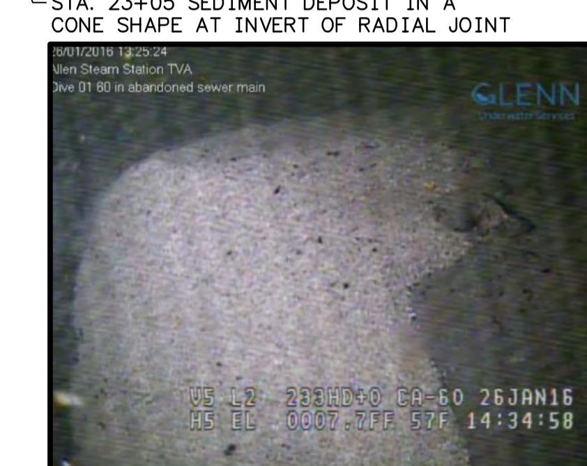
STA. 23+05 SEDIMENT DEPOSIT IN A CONE SHAPE AT INVERT OF RADIAL JOINT
