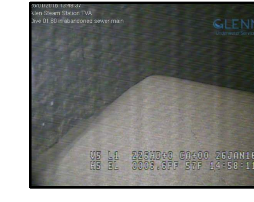
STA. 28+10 SEDIMENT DEPOSIT IN A CONE SHAPE AT INVERT OF RADIAL JOINT
