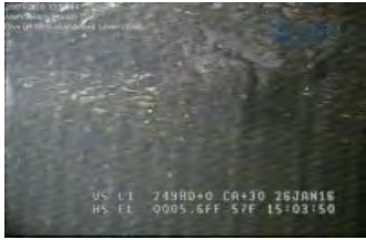
825 ft from manway 17 debris hanging from crown of pipe C1.jpg
