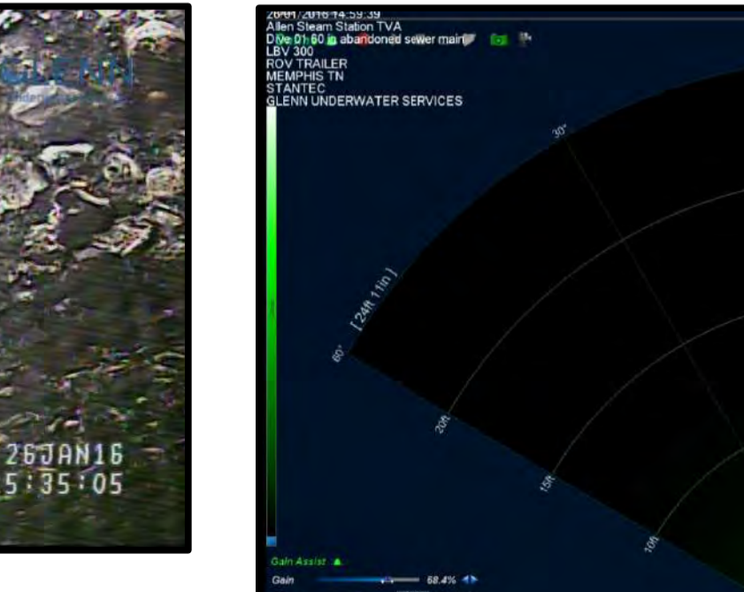
STA. 37+30 DEBRIS IN PIPE UNPASSABLE; INSPECTION ENDED
