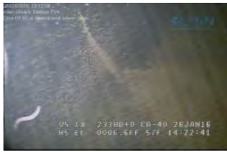
185 ft from manway 17 note debris along wall on oppostie side_C1.jpg
