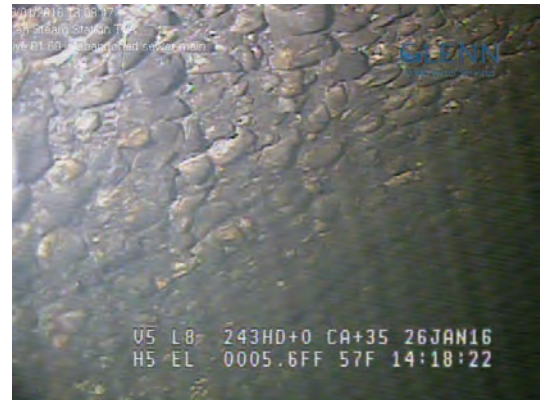
Figure 2 – 155' downstream from manhole No. 17. Example of exposed aggregate.
