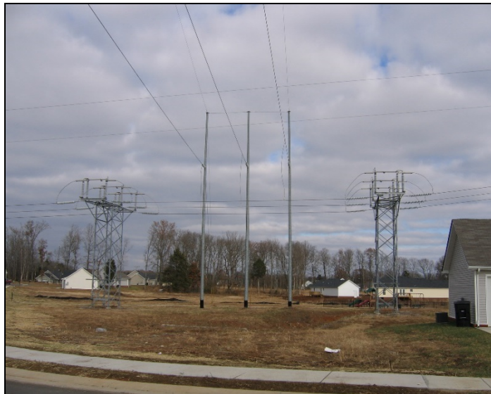
Photo 2-3. Example of switch structures and associated 3-pole transmission structure at a transmission line tap point
